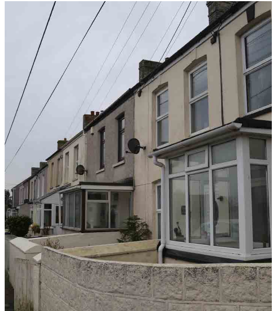
Figure 110: - Erosion of façade character through use of large uPVC porch additions.
