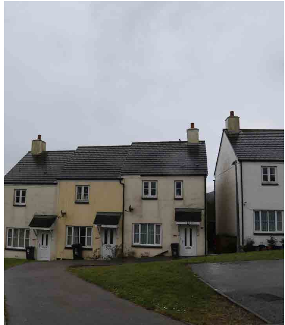
Figure 111: - Rendered façade with severe staining, development lacks materiality variation.
