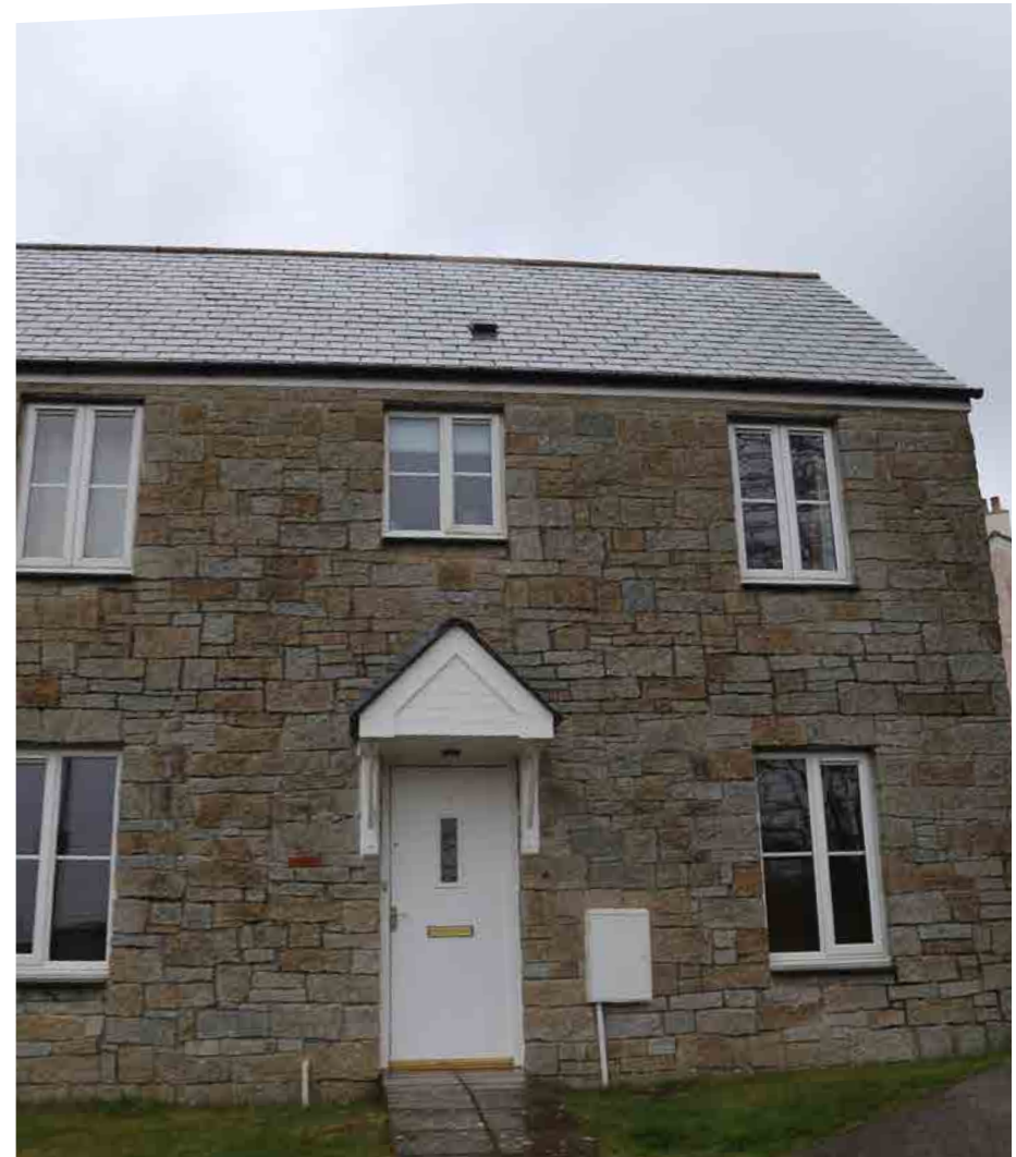
Figure 122: - Poorly placed utilities box impacts building façade.
