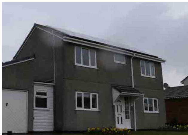
Figure 29: - Full solar array facing east.
