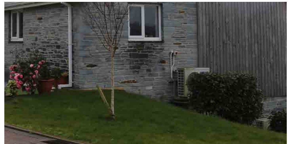
Figure 124: - Air source heat pump, would benefit from subtle enclosure. Vegetation screen growth could foul intake.
