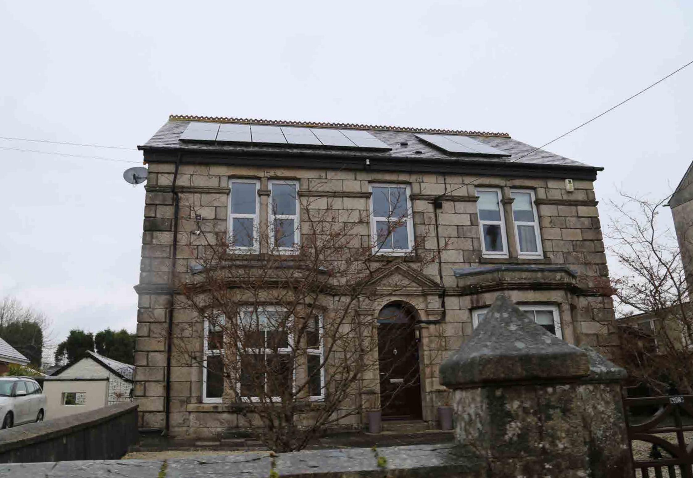
Figure 73: - The best practice for installing PV on heritage dwellings is to keep to secondary elevations. Here PV and cabling detract from the primary elevation.
